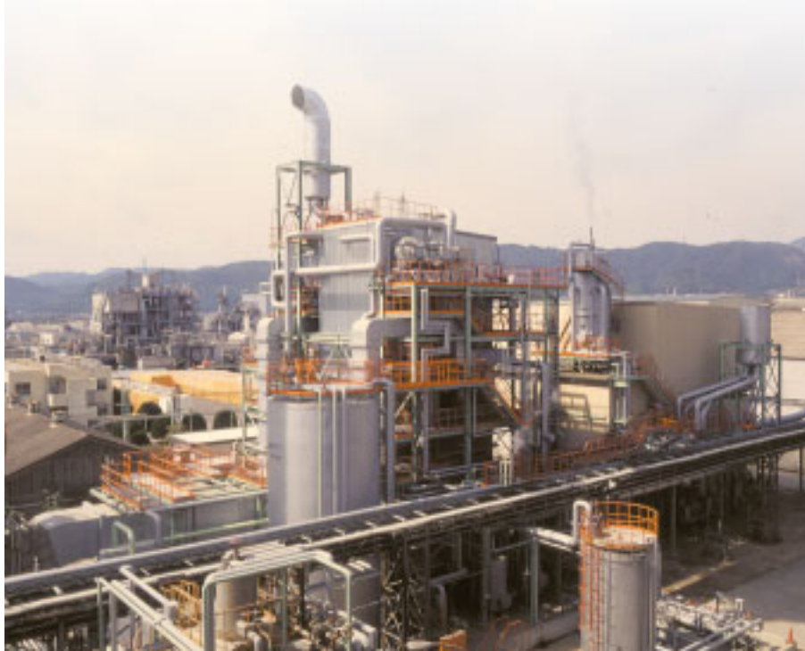
Power generation plant with environmentally friendly boiler (Kawasaki Advanced Clean Combustion) for Japan Paperboard Industries Co., Ltd.
