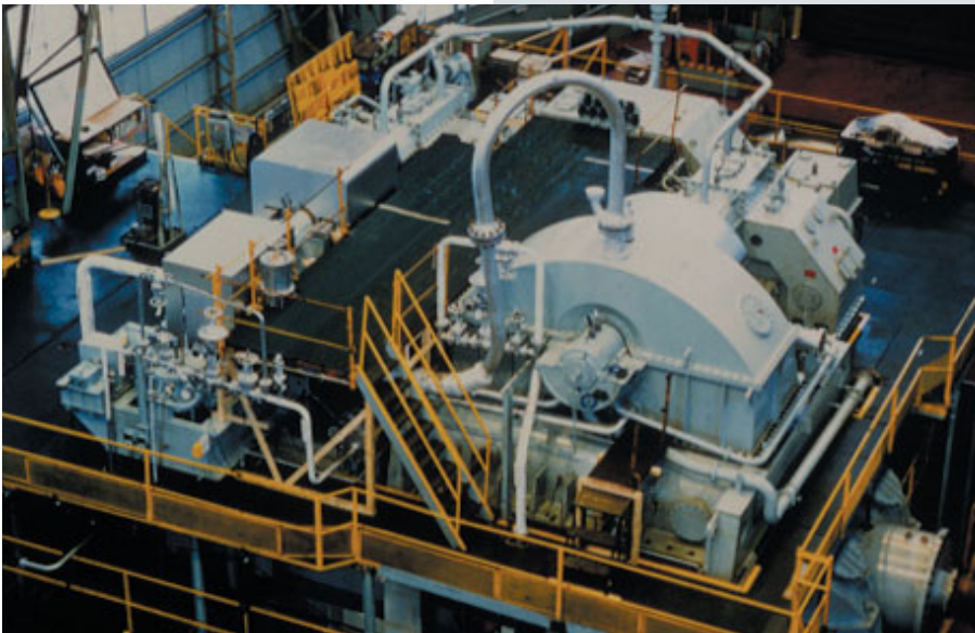
Marine steam turbine (UA-type)
