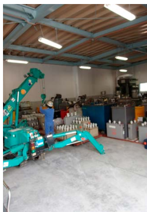
PCB discharge operations
