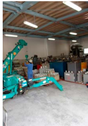
PCB discharge operations
