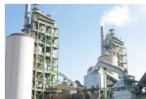
Cement plant waste heat recovery power generation
