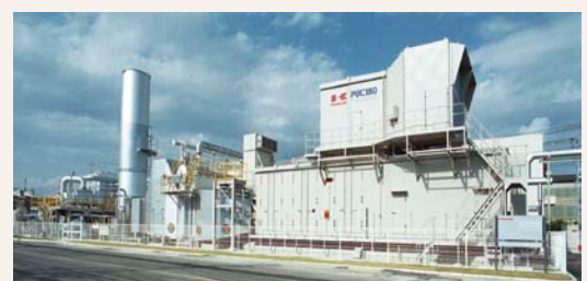
Gas turbine generation system at Akashi Works
