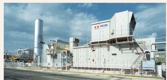
Gas turbine generation system at Akashi Works
