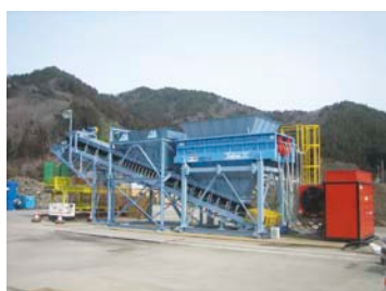
Rubble crushing machine
