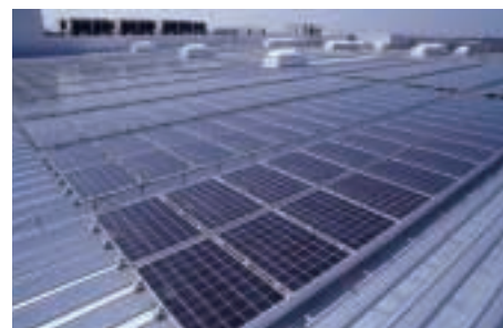
Photovoltaic systems at the Kawasaki Precision Machinery main plant (core parts plant)
