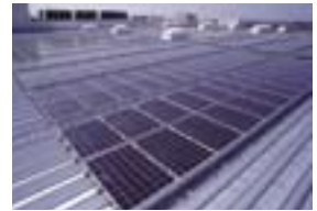
Photovoltaic system at core parts plant
