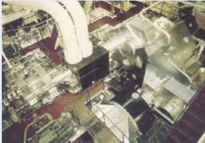
Reheat turbine plant
