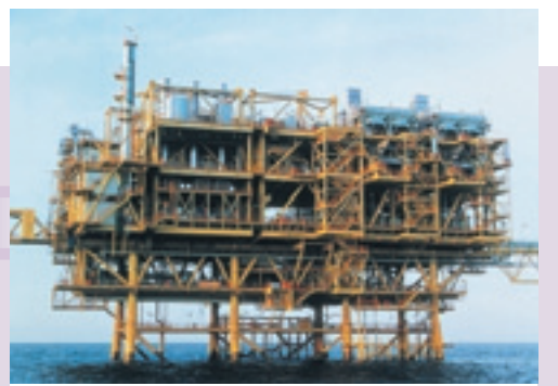
Gas compression module installed offshore
