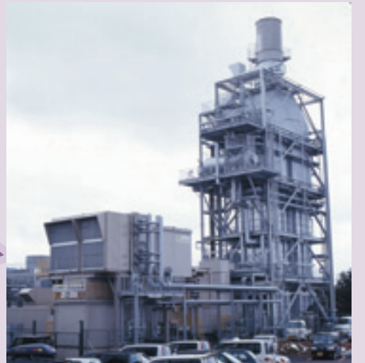
Combined cycle power plant (25 MW) equipped with Kawasaki gas turbine L20A
