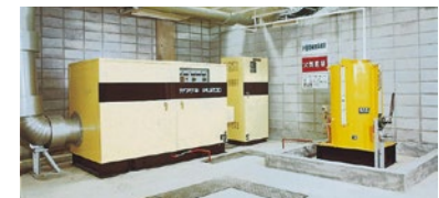
1976 Developed the Kawasaki GPS200 , the first Japan-made gas turbine generator
