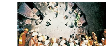
1991 Successful excavation of the Channel Tunnel, linking France and the United Kingdom
