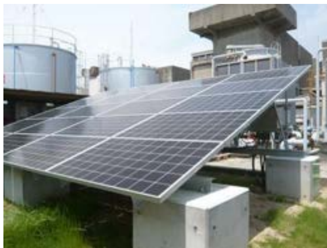
PV panels at the Akashi Works
