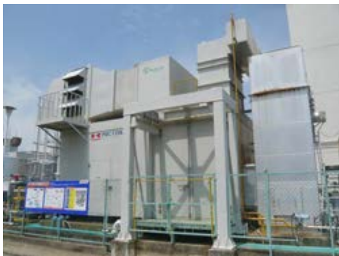
An M1A-17D gas turbine at the Akashi Works
