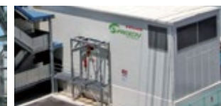
Figure 12: Onsite power generation facilities at Kobe Works (gas engine)
