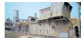
Figure 11: Onsite power generation facilities at Akashi Works (gas turbine)
