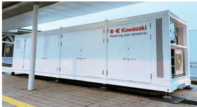
Fig. 2 Example container installation
