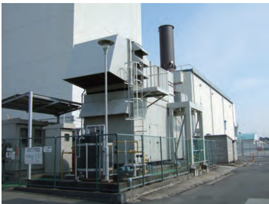
Fig. 9 Electric power plant at Akashi Works
