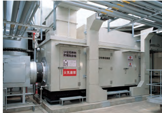
Fig. 6 Gas turbine of dual-fuel specification
