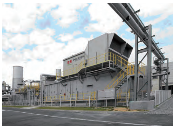
Fig. 5 Akashi Works Energy Center
