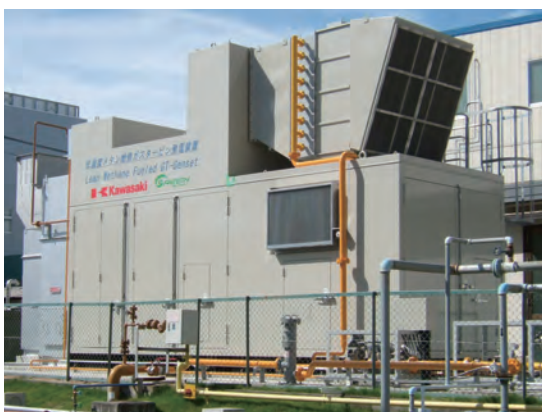
Fig. 5 Lean methane-fueled gas turbine generator set
