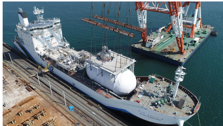
Installation of liquefied hydrogen cargo tank on the world's first liquefied hydrogen carrier
