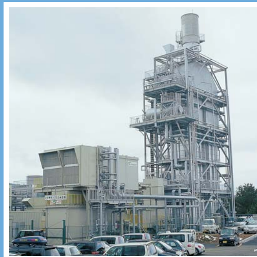
25 MW combined cycle power plant with L20A gas turbine for Daihatsu Co., Ltd.
