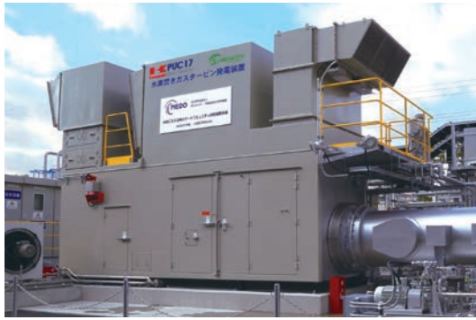
図10 水素-天然ガス燃料混合比自在型の熱電併給設備 Fig.10 Cogeneration facility with flexibility in the fuel mixing ratio of hydrogen to natural gas
