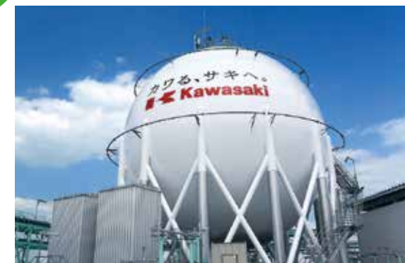
Liquefied hydrogen storage tank at Hy touch Kobe
